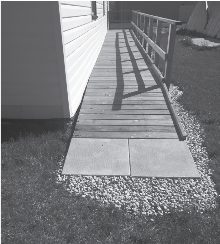
Work continues at the fairgrounds with a new hand-capped ramp to the Heritage Hall. Thank you to Rob Munro, Bill Cameron, Brandon & Jarrett Ritchie.
